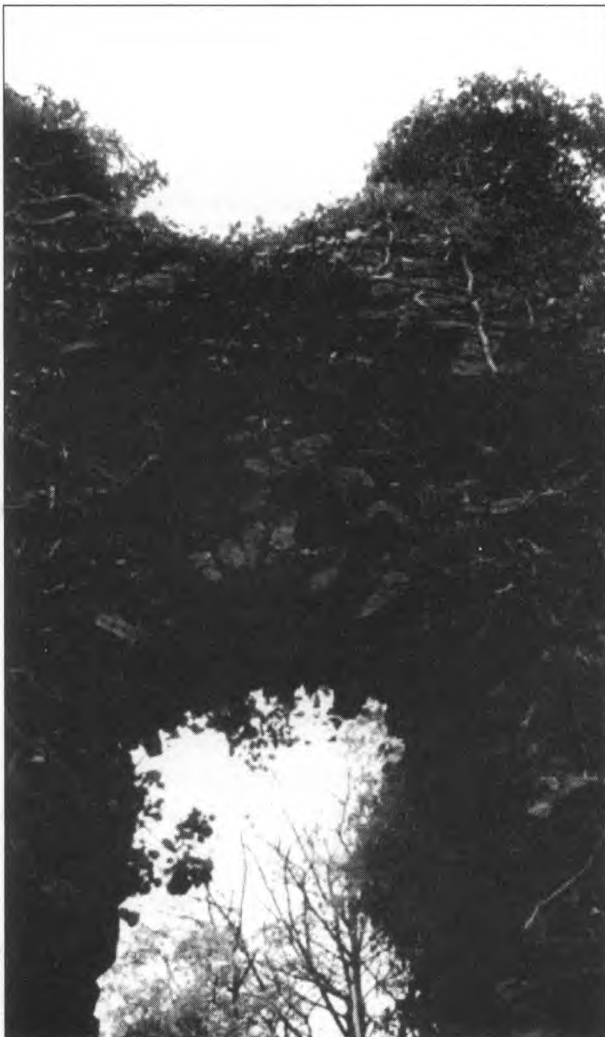
Archway at the castle before (left) and after (right) emergency consolidation work by Cadw.
